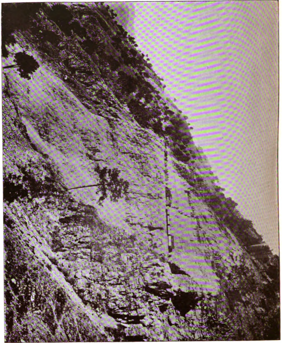
THE SIMLA KAIKA RAILWAY. (A HILL SLIP AND BREAST WALL).
